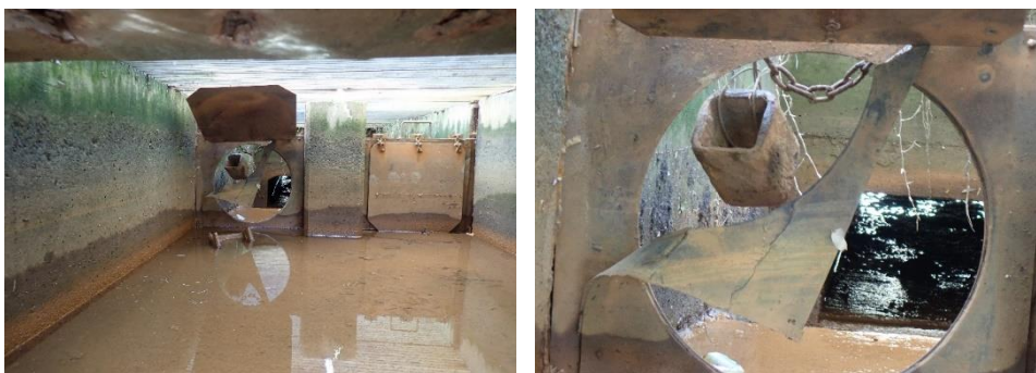
Figure 12 (left) in and outflows can be regulated with floodgates; (right) the floodgates are rusty and have fallen into disrepair
