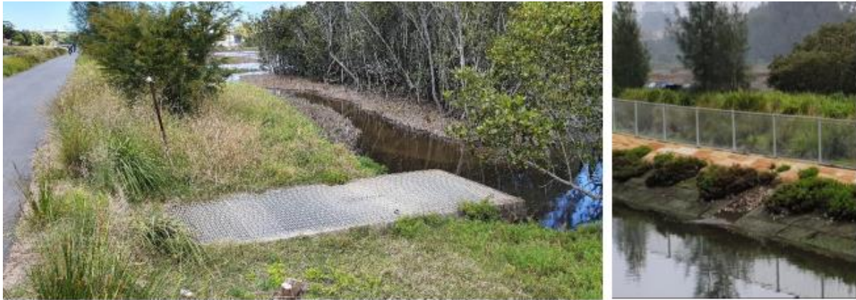
Figure 7 Existing inlet/outlet structure, at wetlands (L), grate over culvert on Powells Creek side (R)
