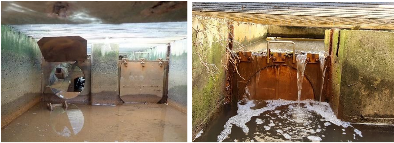
Figure 13 Internal view of inlet/outlet structure, looking from wetland side when drained (L), looking from Powells Creek side with water held in the wetlands (R)
