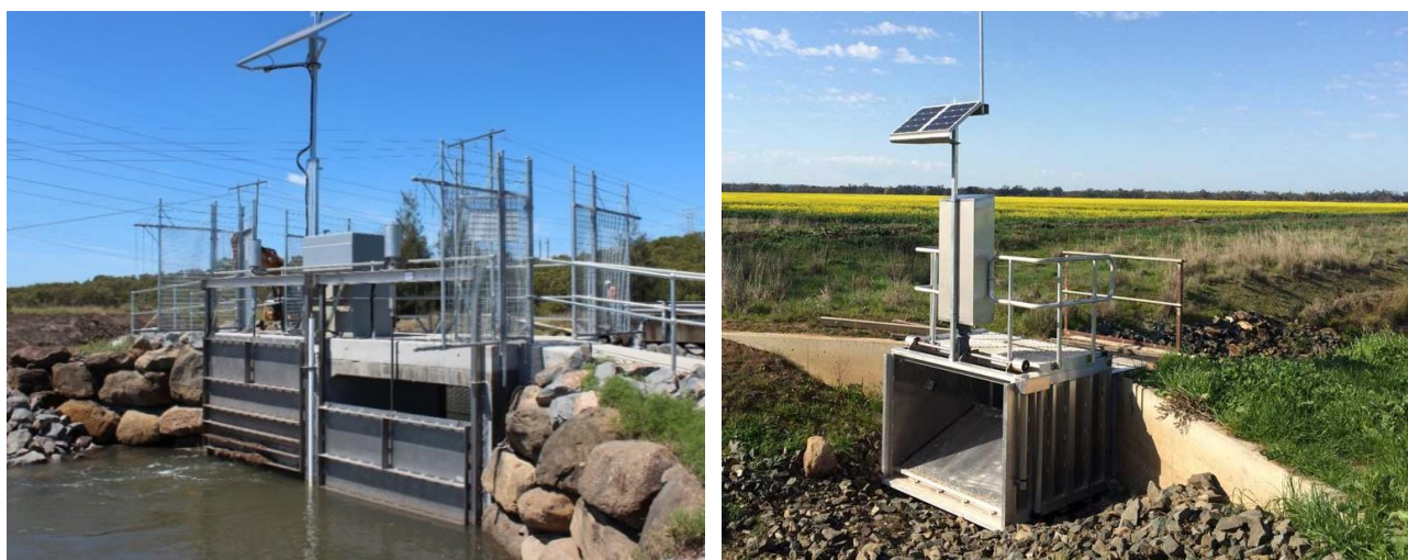
Figure 24 Example of automatic water control gate systems
