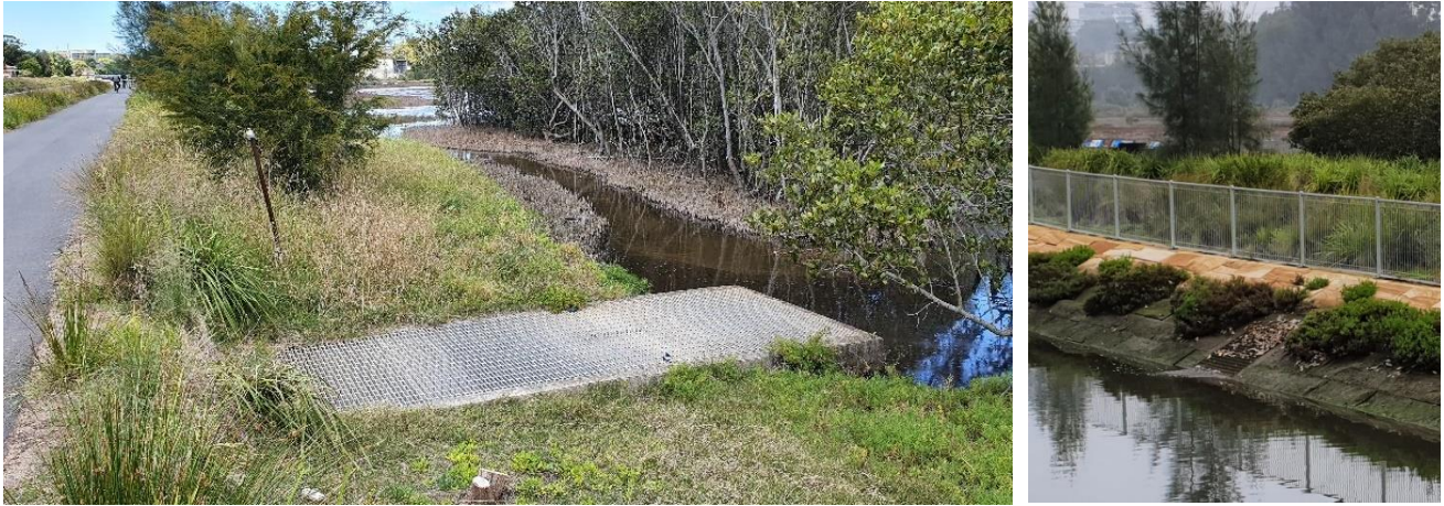
Figure 11 Existing inlet/outlet structure, at wetlands (L), grate over culvert on Powells Creek side (R)
